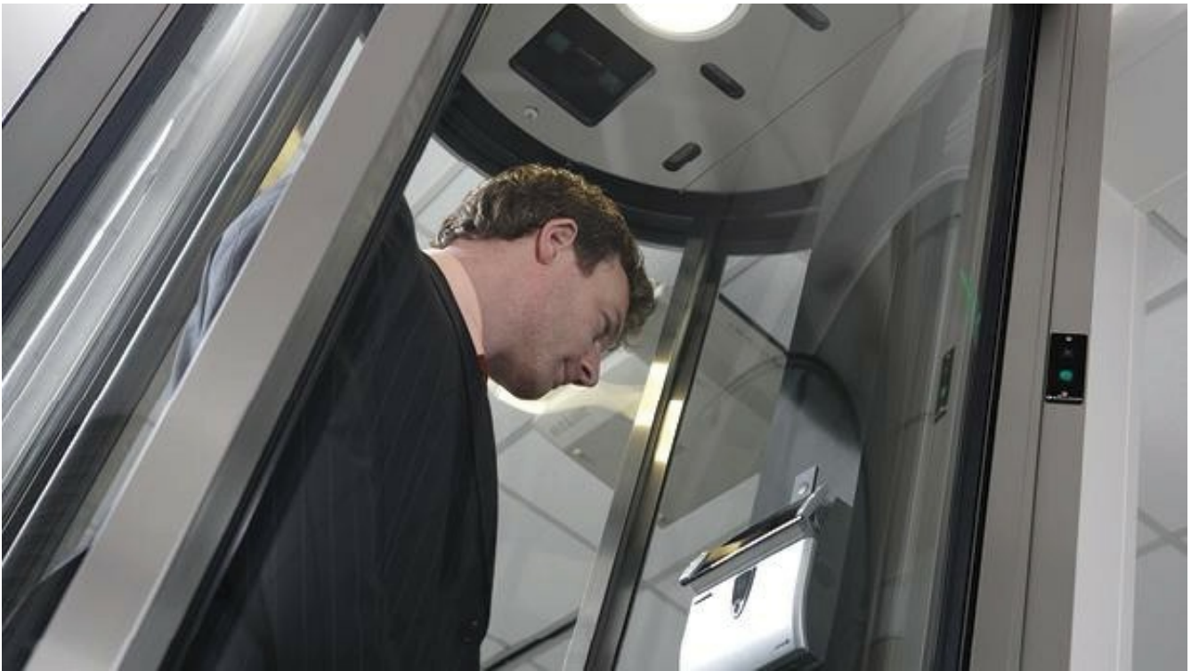
Figure 3.51 - A Secure Portal allows only one person in at a time and will only open the inner door once the outer door is closed.
