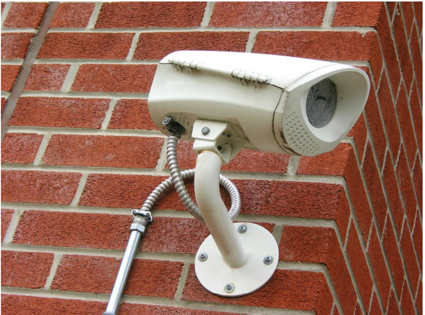
Figure 7.15 – A Wall-Mounted Camera
