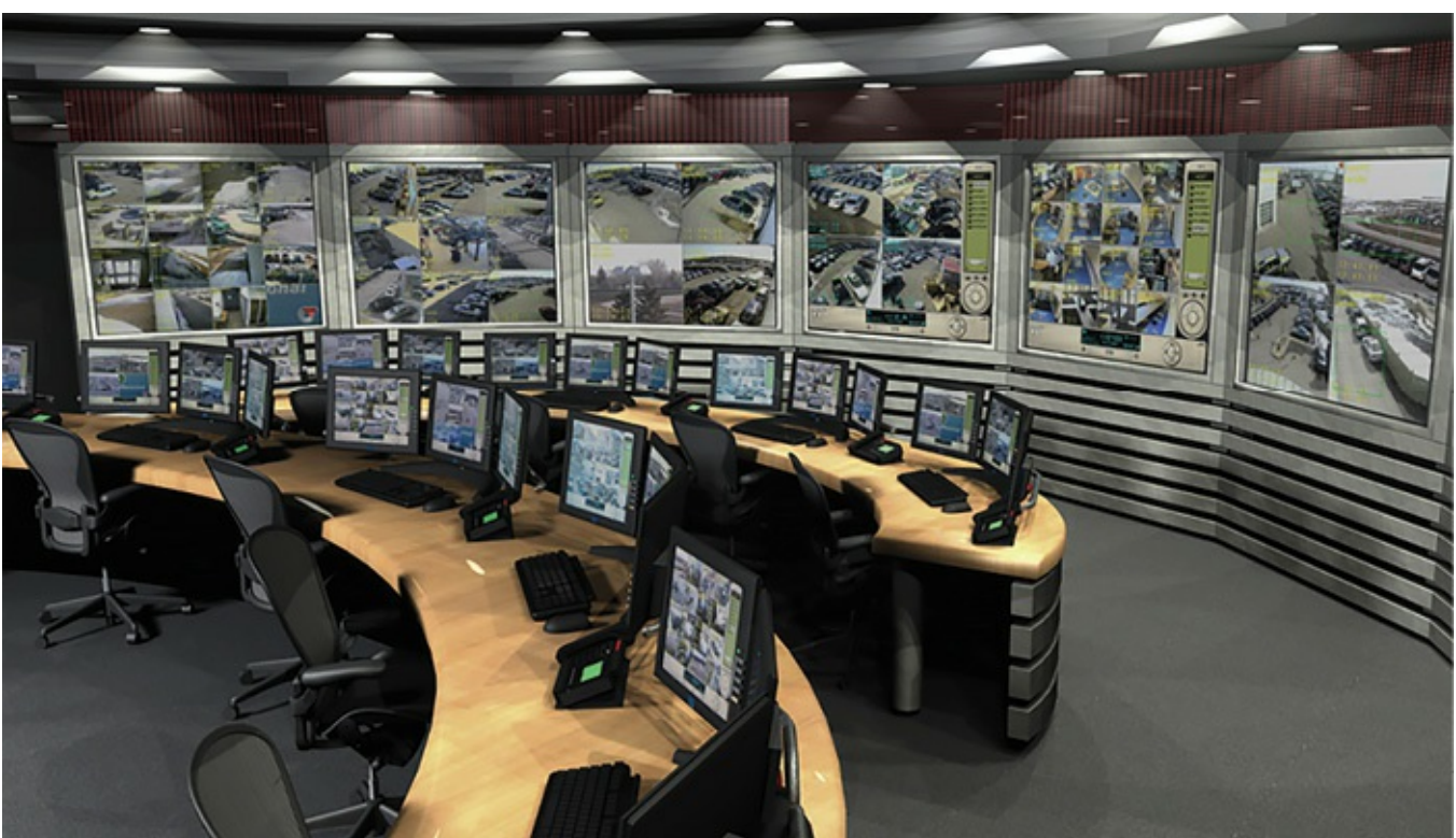
Figure 7.20 – The central center, also known as the security console center, security control center, or dispatch center, is an area that serves as a central monitoring and assessment space for access control, CCTV, and intrusion detection systems.
