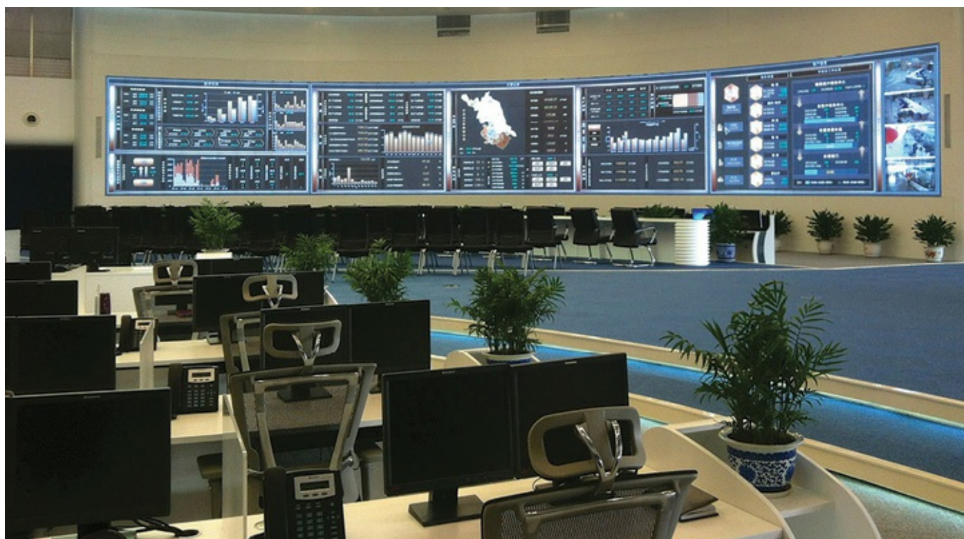
Figure 7.19 – Large format displays in a power facility
