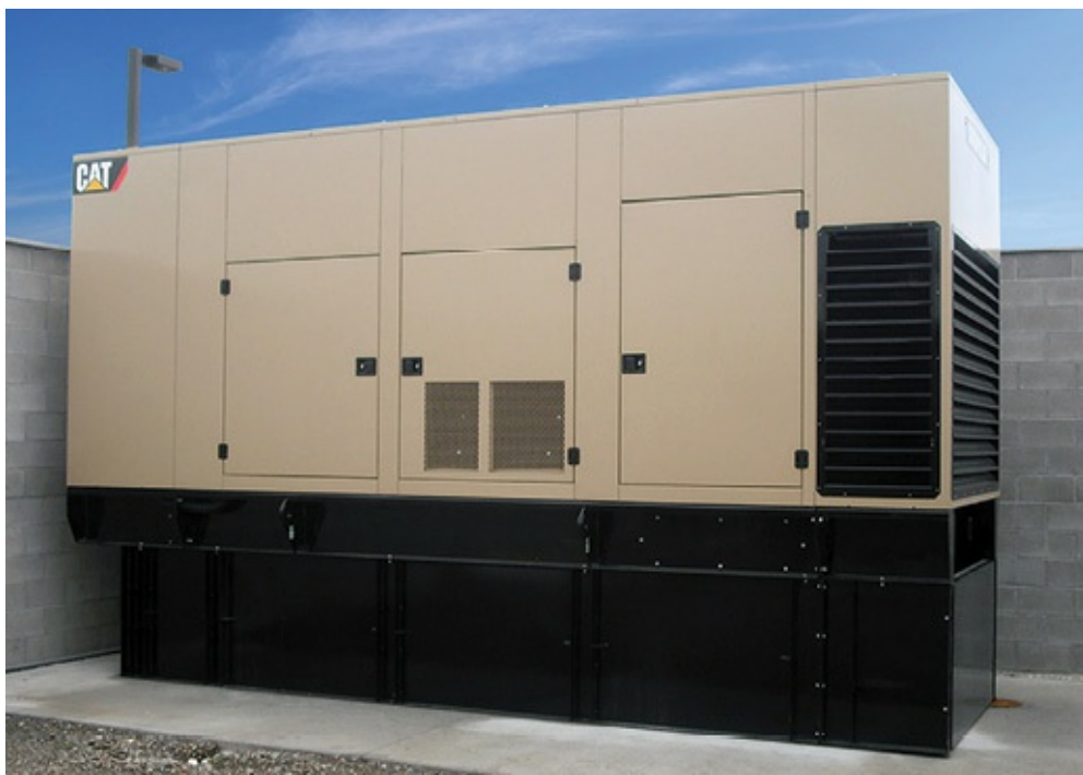
Figure 3.52 - A Backup Generator is activated automatically in the event of a utility failure by the transfer switch.
